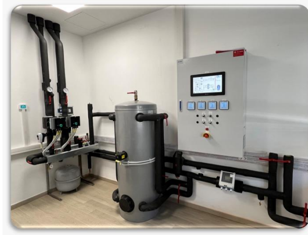
Figure 10: Laboratory setup with air/water heat pump on FSB
