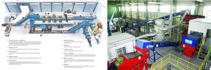
Figure 2. Installation for separation of the company "Recycling" Bulgaria. The Ekobulpak plant has a total area of 11,000 m 2 (photo: Alyosha Dimitrov)
